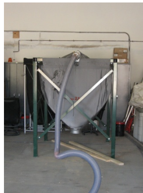
... blows pellets to an indoor flexible bag silo which can store 1- 10 tons...
